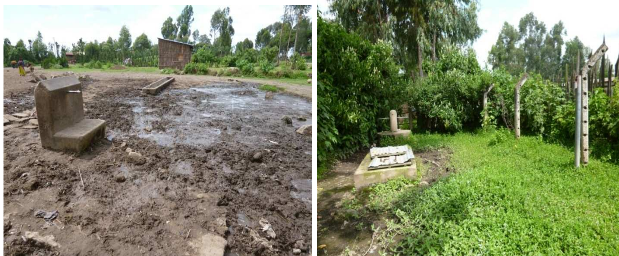
Figure 4-2 Non-functional water supply schemes in the R-WASH intervention Kebeles
