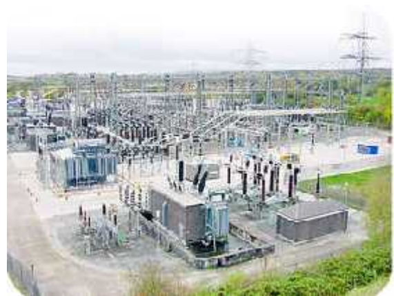
Substation. Source: www.innovative.co,nz
