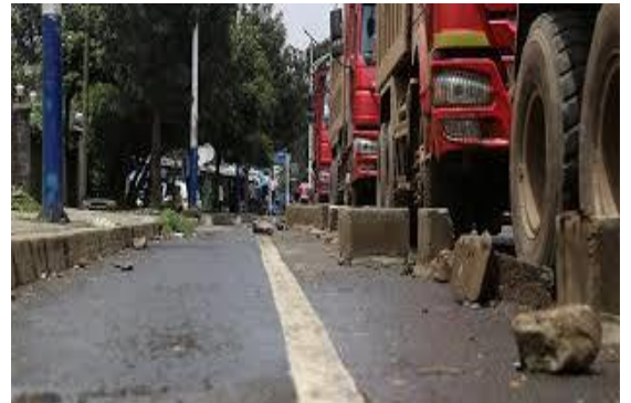
Figure 1.5: Damaging cycling infrastructures.
