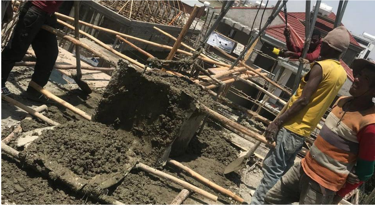
Fig: - 4.9 Wastage of concrete due to poor transport
