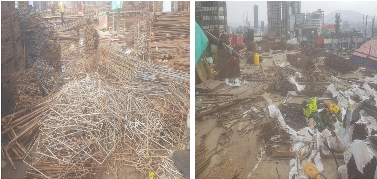
Figure: - 4.4 wastage of steel reinforcement bar due to non-optimized cutting of bars and design change
