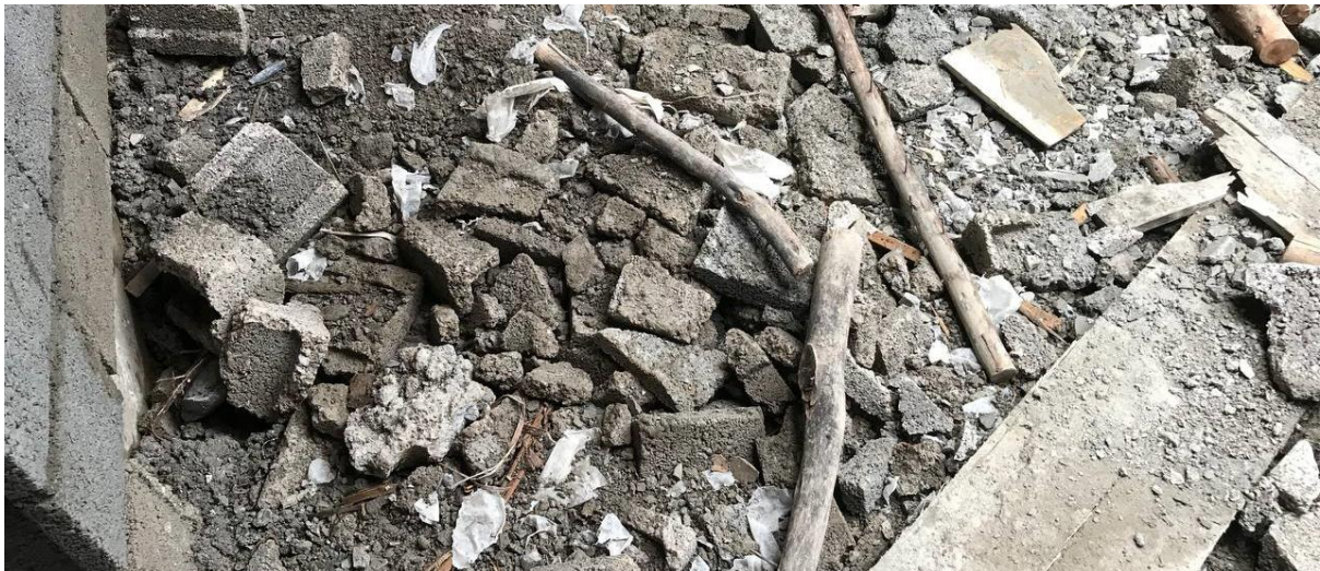
Fig: - 4.13 Wastage of cement mortar due to chiseling and design change on building sites
