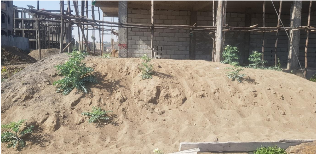
Fig: - 4.6 Poor handling of sand onsite
