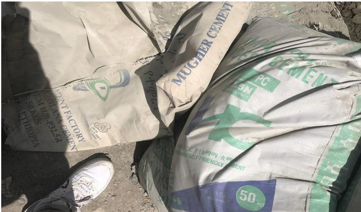
Fig: - 4.10 Wastage of cement due to poor handling lack of control and poor storage
