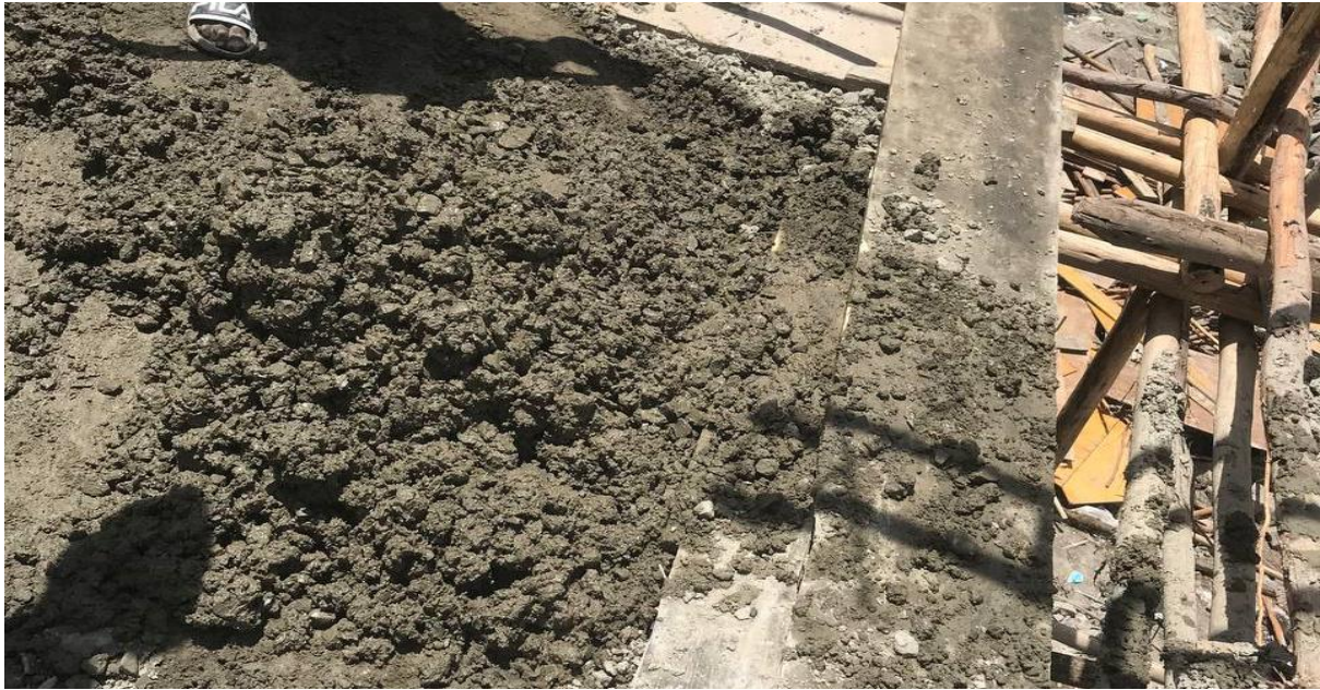
Fig 4.12 Mixing of mortar greater than the required
