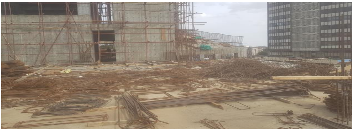
Figure: - 4.5 Poor handling of steel reinforcement bar on building construction site
