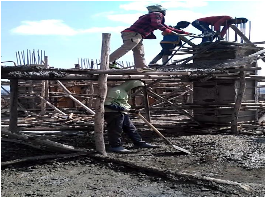
Figure 4.3 Improper transporting of concrete
