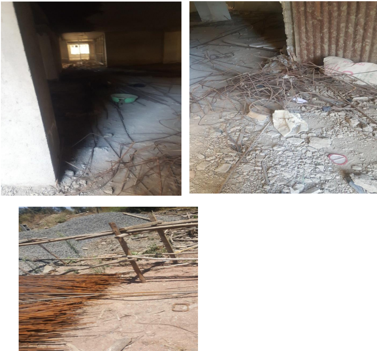
Figure 4.1 Improper handling of Reinforcements bar
