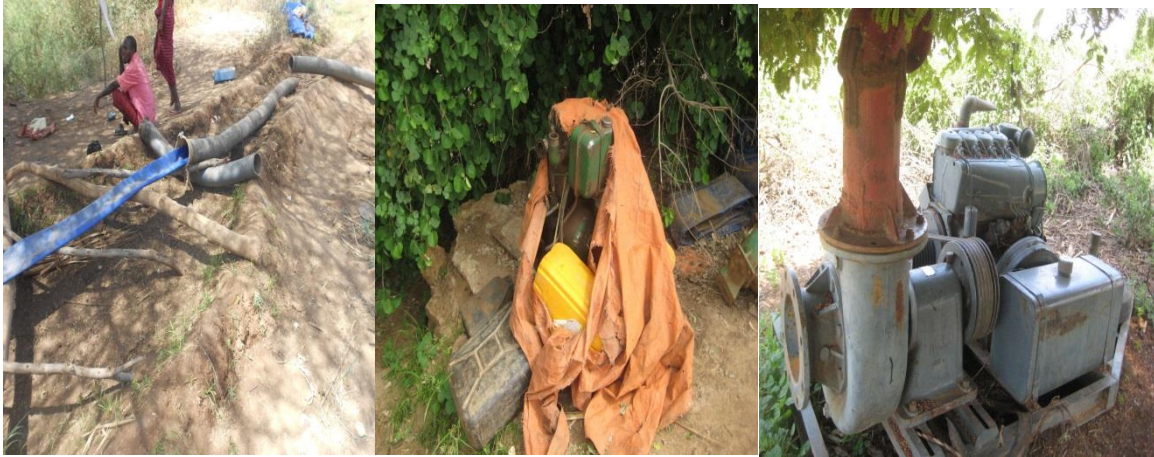
Figure 13: Broken motor pump at Dasheg kebele, Dolo Bay woreda
