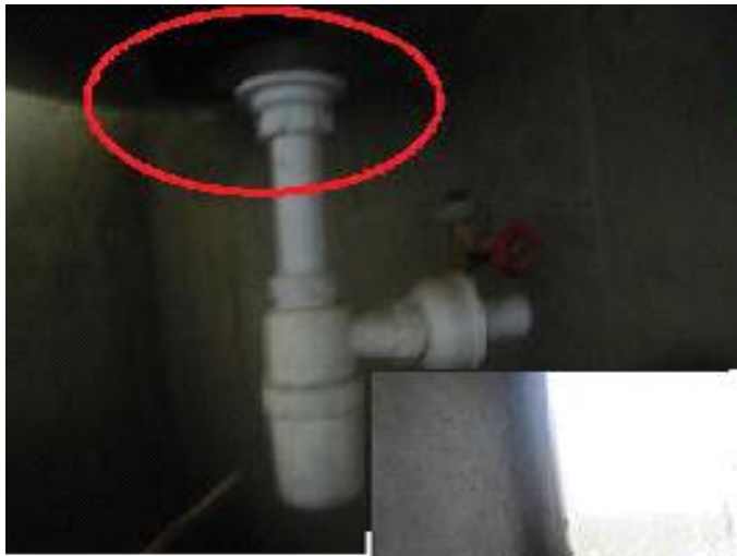
Improper fixing of kitchen-sink fitting
