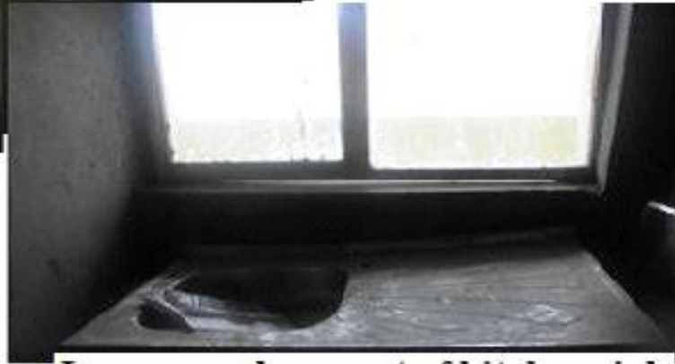
Improper placement of kitchen sink
